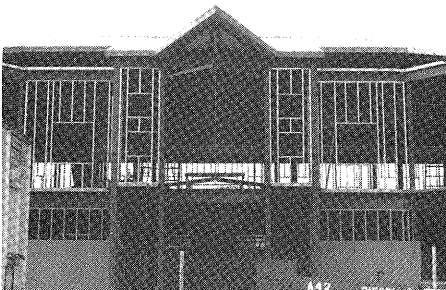
Framework in place for main entrance area. Photograph by John H. Talley.
