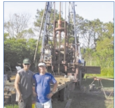
Drillers Manuel Canabal and Gene Cobbs III and the Mobile truck-mounted drilling rig.
